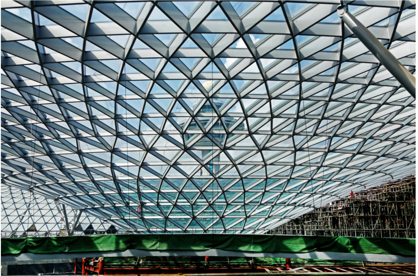
The iconic façade of Jewel Changi Airport is being built in its last phase of construction. PHOTO: LIANHE ZAOBAO
